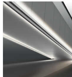
LED cove lighting Side and soffit cladding
