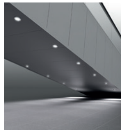
Soffit LED spot cladding lighting
